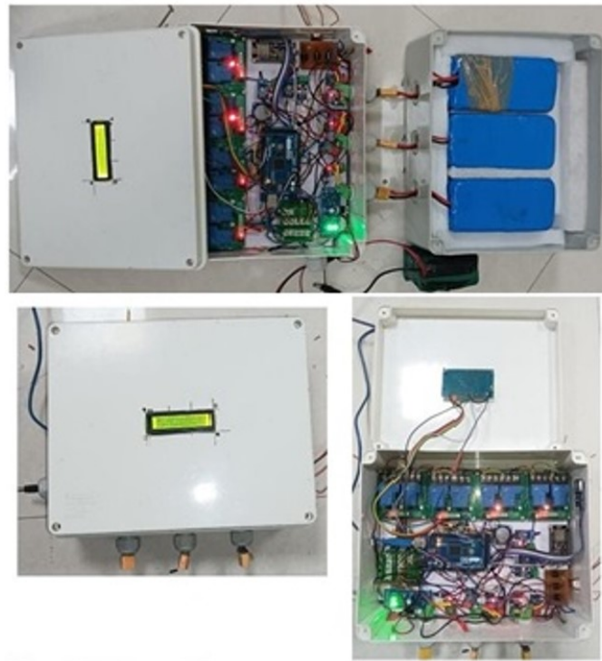
Fig. 4.1: BMS and SOC connected to Primary Battery, Solar battery, and Turbine battery
