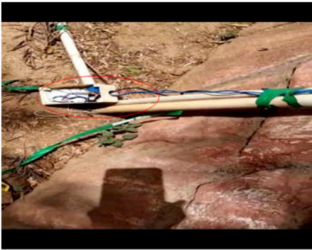
Fig. 4.4: Street Light System Prototype installed at ITM Gwalior Sithauli Campus
