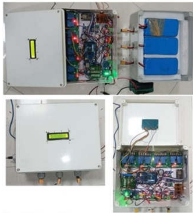
Fig. 4.1: BMS and SOC connected to Primary Battery, Solar battery, and Turbine battery
