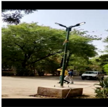
Fig. 4.6: The process is repeated for another moving objects (human presence) the lights TURNED ON in this picture, Sithauli Campus at ITM Gwalior
